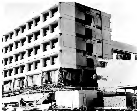
Photo 22. Medical Treatment Building, toward the southeast corner. Note overturned stair tower at right, broken columns, and collapsed ground story under landscaping. Los Angeles County Fire Department photo.
